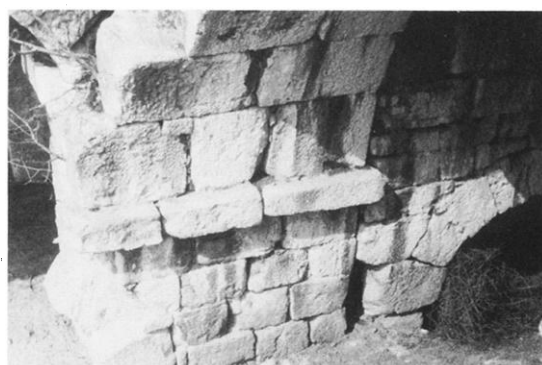
(d) Middle pier of vaulting, showing join of first phase (with cornice) and second phase (with water channel).
